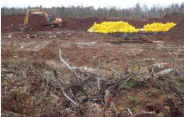
Photo 12: Current Phase 2 cell with yellow bagged asbestos waste waiting to be placed in excavated cell.
