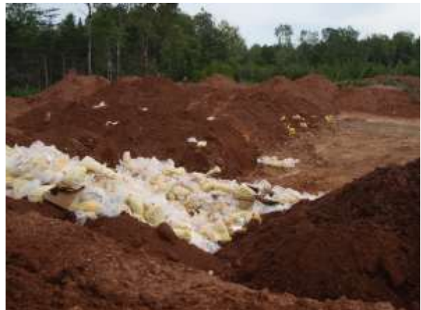
Photo 13: Bagged asbestos waste in current Phase 2 disposal cell. Waste is covered with a minimum 0.25m of soil within 24hrs of delivery.
